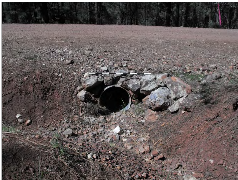
Photograph 6. Feature 49, an example of Type 1B CMP with a dry laid masonry headwall, facing north.
