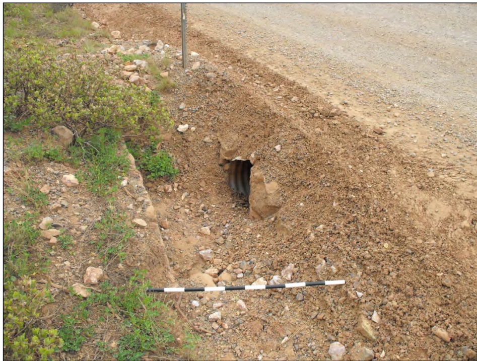
Photograph 7. Feature 297, an example of a Type 1C feature with a partially destroyed headwall, facing southeast.
