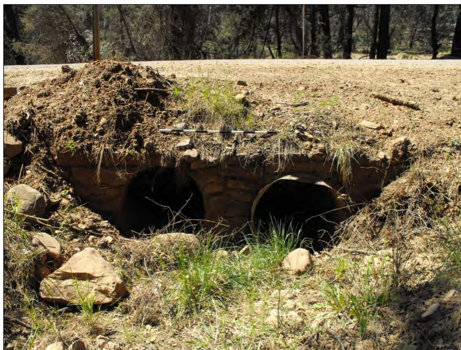
Photograph 3. Feature 149, a mortared Type 1B feature with a double CMP, facing northwest.
